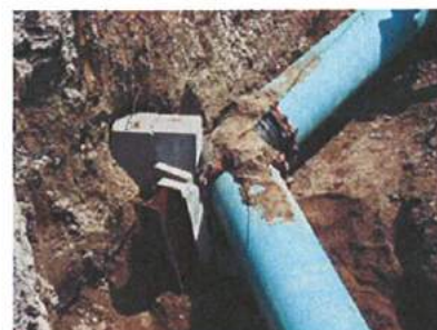
Plastic pipe eases worry about rusting, which consumes the chlorine residual that kills fungal growth in a water system, and "red water" complaints from customers.
