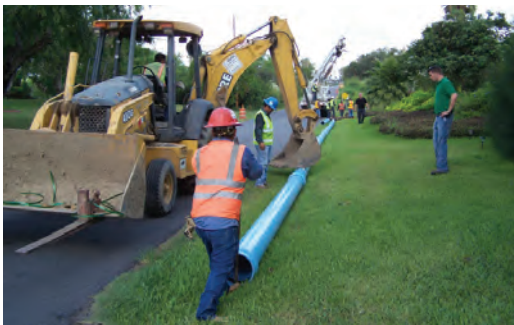
Figure 10: The backhoe's bucket center loads the previously installed length of pipe to keep it from moving while the new joint is being assembled
